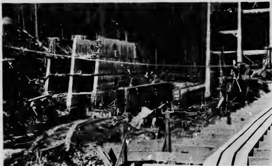
Vancouver Island Power Company Limited. Upstream showing portion of Jordan River Dam in river bed, in course of construction.
